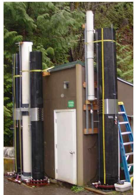
Slow sand pilot filter columns
